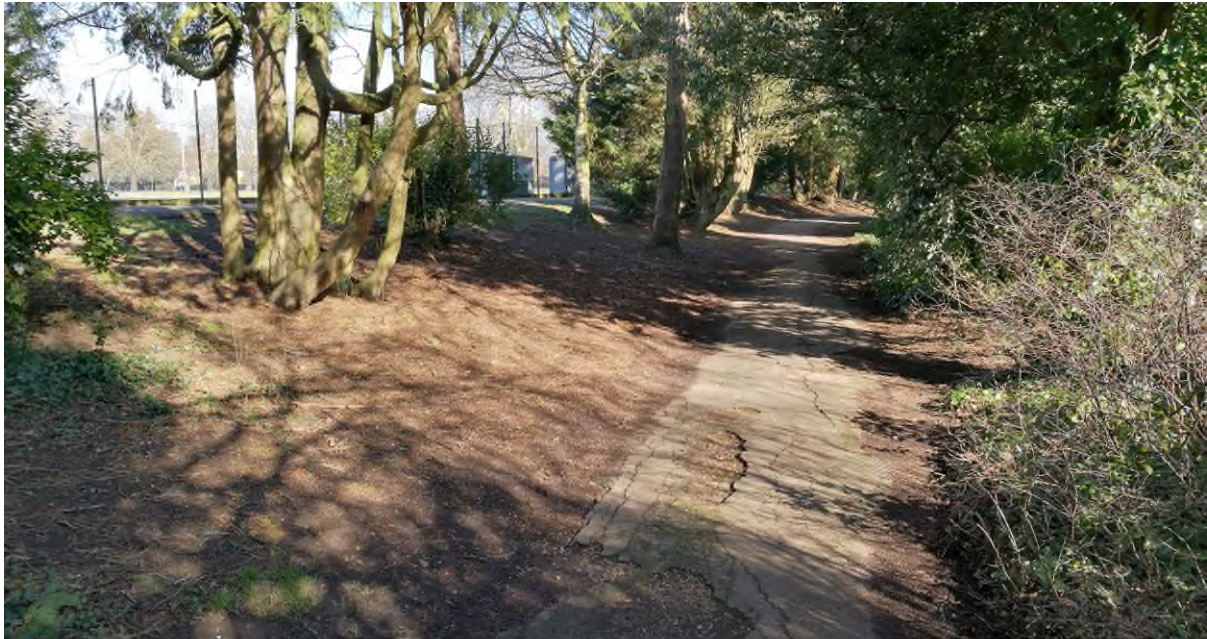
Path on the eastern perimeter with breaking surface and little horticultural interest
