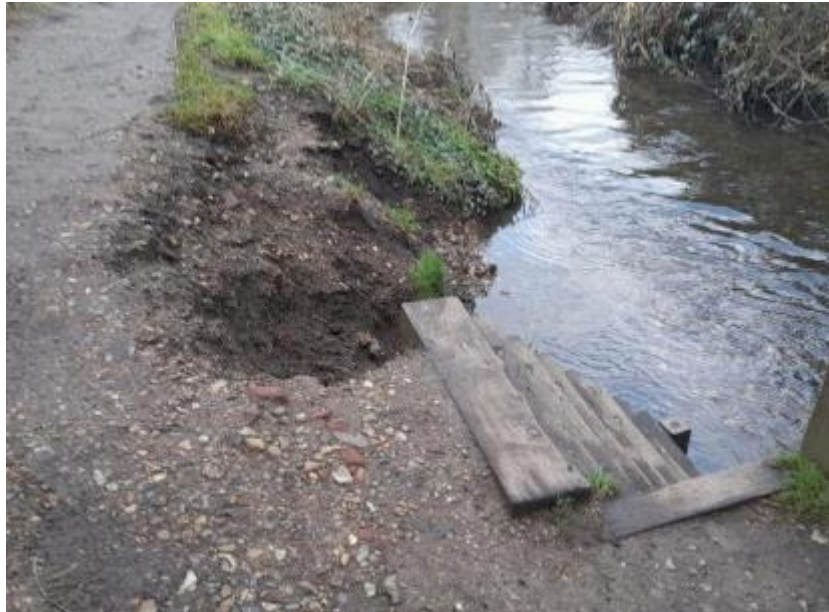
Erosion around dog steps installed on the River Ver.
