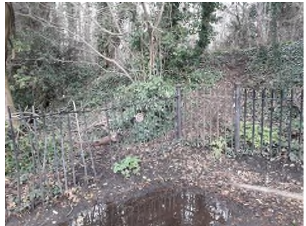
Dilapidated fencing at entrance from Abbey Mill Lane
