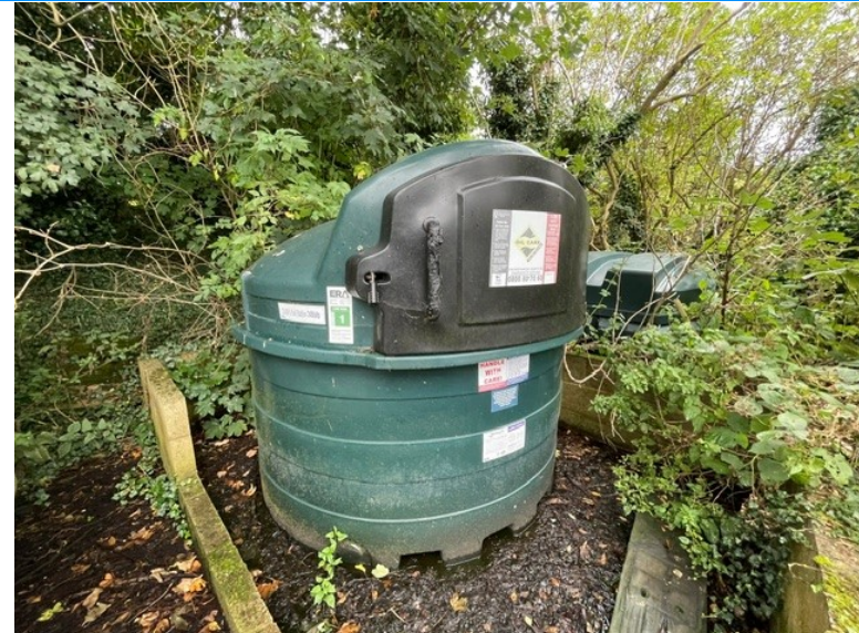
22. Tanks shown on concrete plinth.
