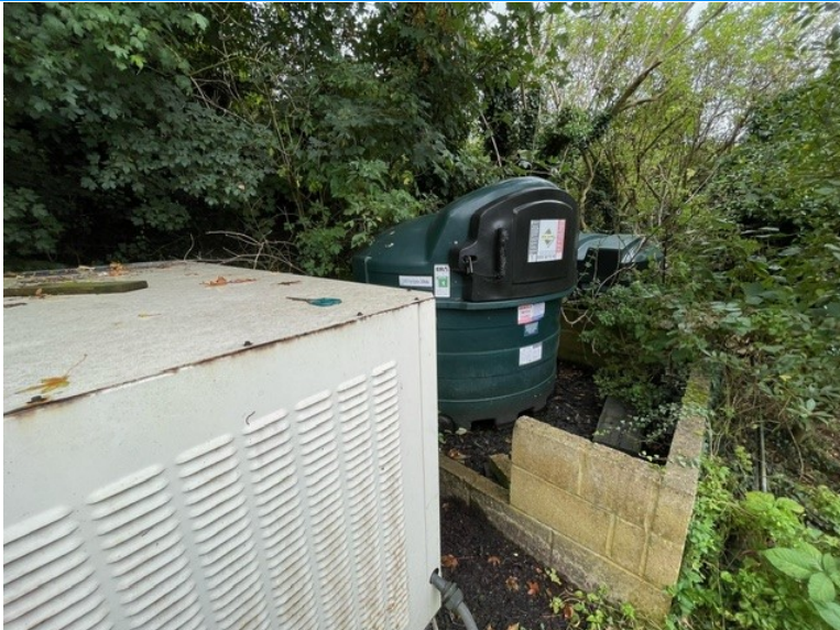
21. Generator and tanks behind the indoor riding arean.
